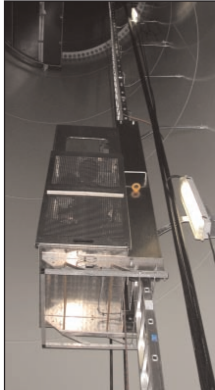
Worm's eye view of wind turbine tower hoist showing how support frame and undercarriage are secured to metal ladder.
