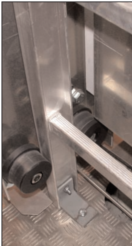
Base of emergency ladder/guide rails showing securement to metal landing. Note guide wheels attached to cage frame that hold and stabilize the cage along both sides of the ladder.
